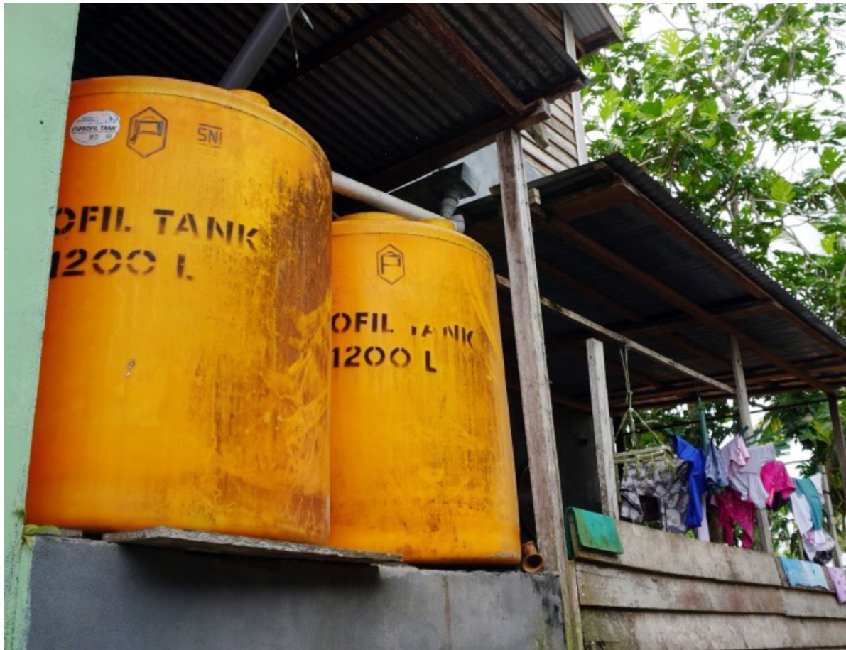
Figure 18. Tank profile for collecting rainwater behind Erni's house, resident of Tanjung, Tanah Kuning.
